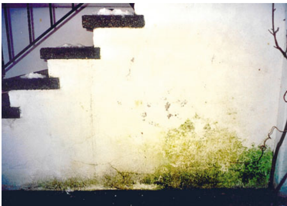
Fig. 14.19 Growth of algae on a painted facade
