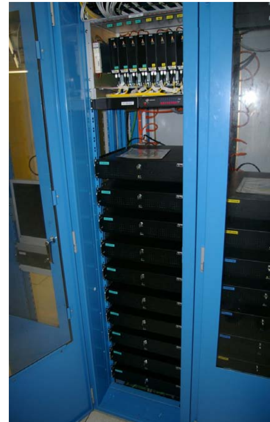
Gateway PCs installed in an LHC access point
