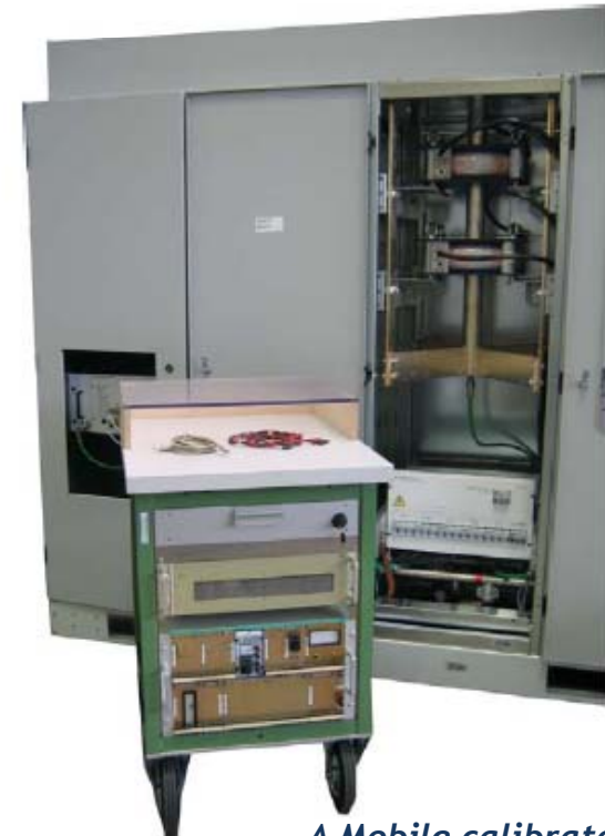
A Mobile calibrator used to calibrate a 6kA converter
