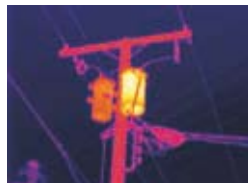
Overheating pole transformer
