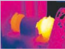
Overheating bearing cap
