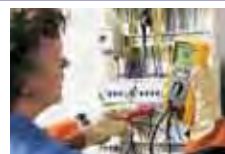
Insulation test at a distribution panel
