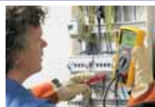
Insulation test at a distribution panel
