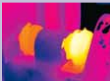
Overheating bearing cap
