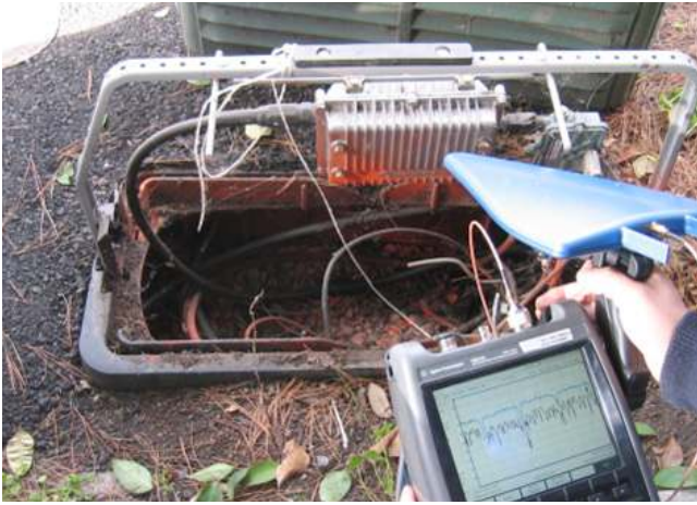
Figure 1a. FieldFox connected to a directional antenna for locating a source of radio interference
