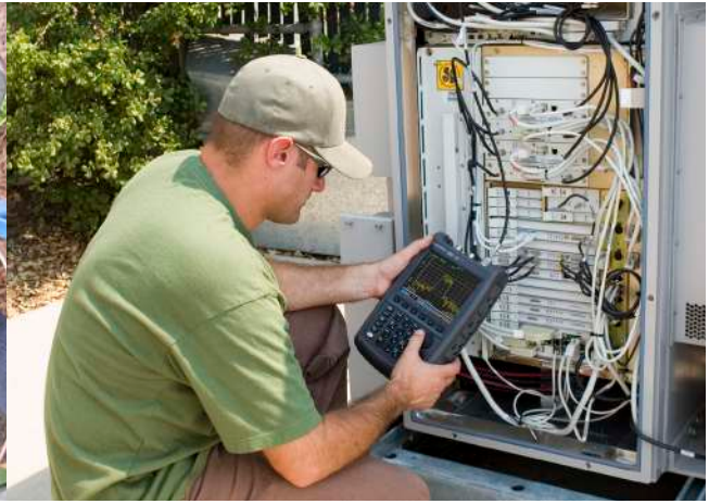
Figure 1b. FieldFox directly connected to a feeder line on a wireless communication system
