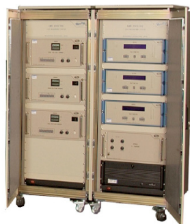
Control Cabinet with Components
